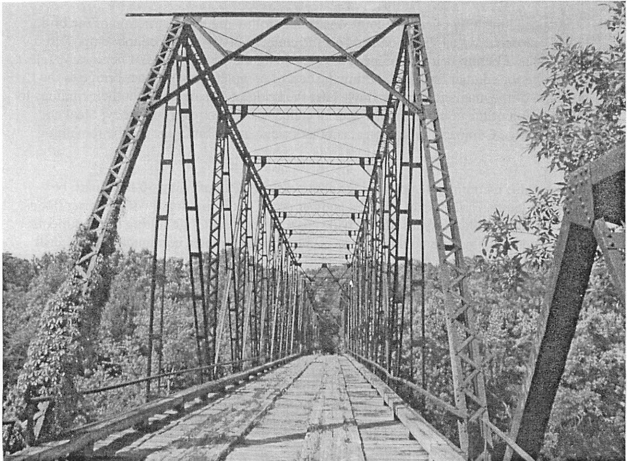
LAYCOCK BRIDGE, CANEY FORK RIVER BETTY'S BEND ROAD PRIOR TO DEMOLITION OF BRIDGE IN 2008
