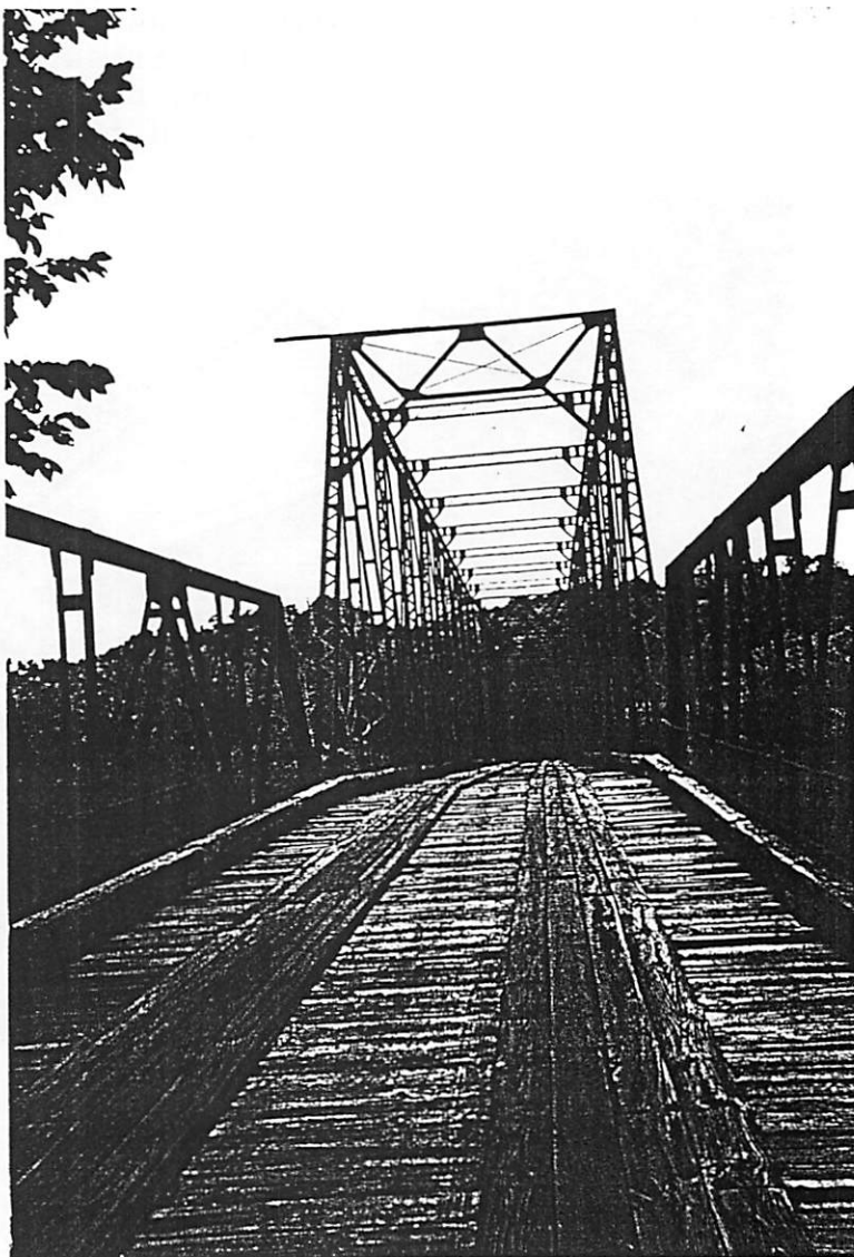
PRECARIOUS OLD LAYCOCK BRIDGE
